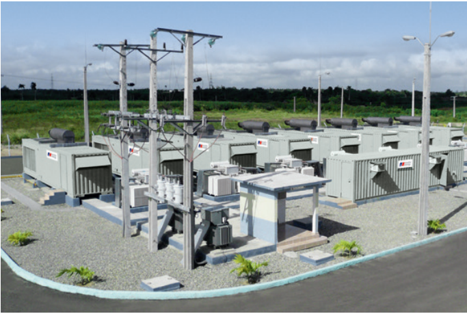
Power Station, Caribbean
