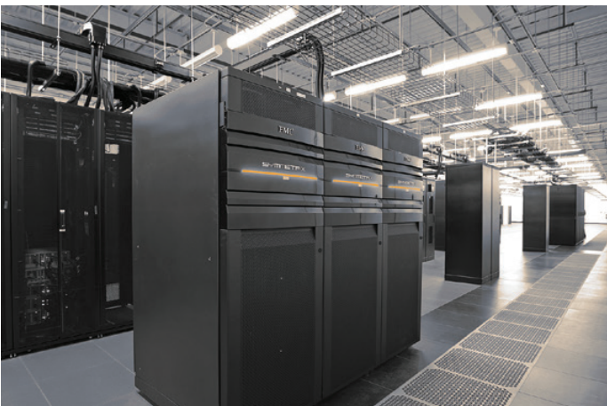
Data Center, Power Loft, USA
